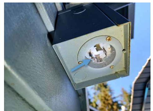
Paint noted at Rear/Left Side outlet
