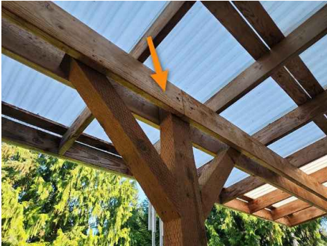
Non-standard framing connection at post to beam
