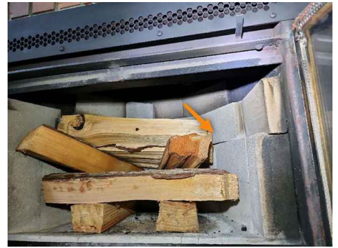
Fire bricks appear to be covering steel firebox lining
