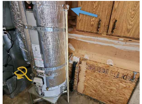
TPR appears to drain to garage slab
