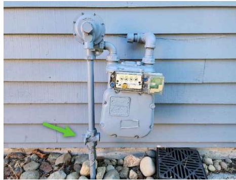
Meter at Left Side
