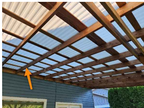
Rafters appear undersized
