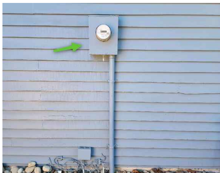
Meter at Left Side
