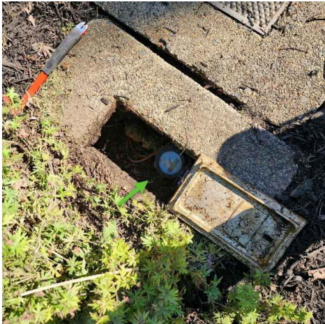
Meter at front
