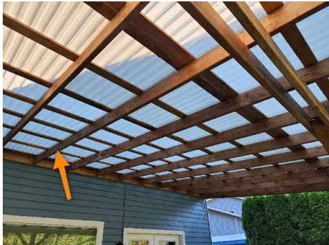
Rafters appear undersized
