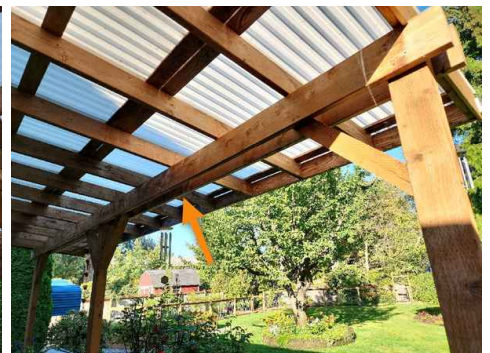
Beam appears undersized
