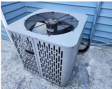
Condensor at Left Side
