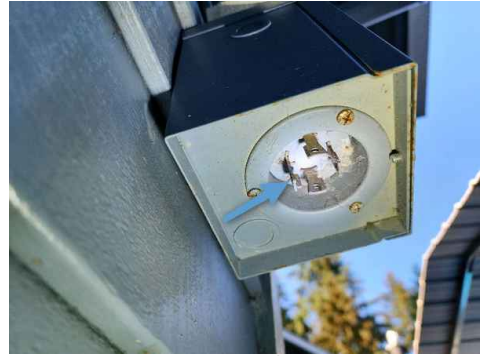
Paint noted at Rear/Left Side outlet
