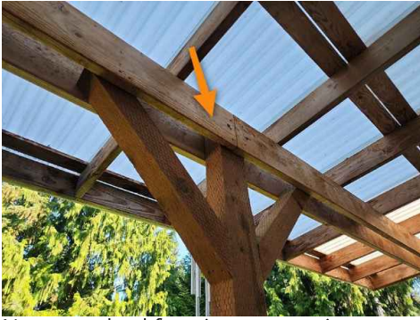
Non-standard framing connection at post to beam
