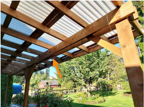
Beam appears undersized
